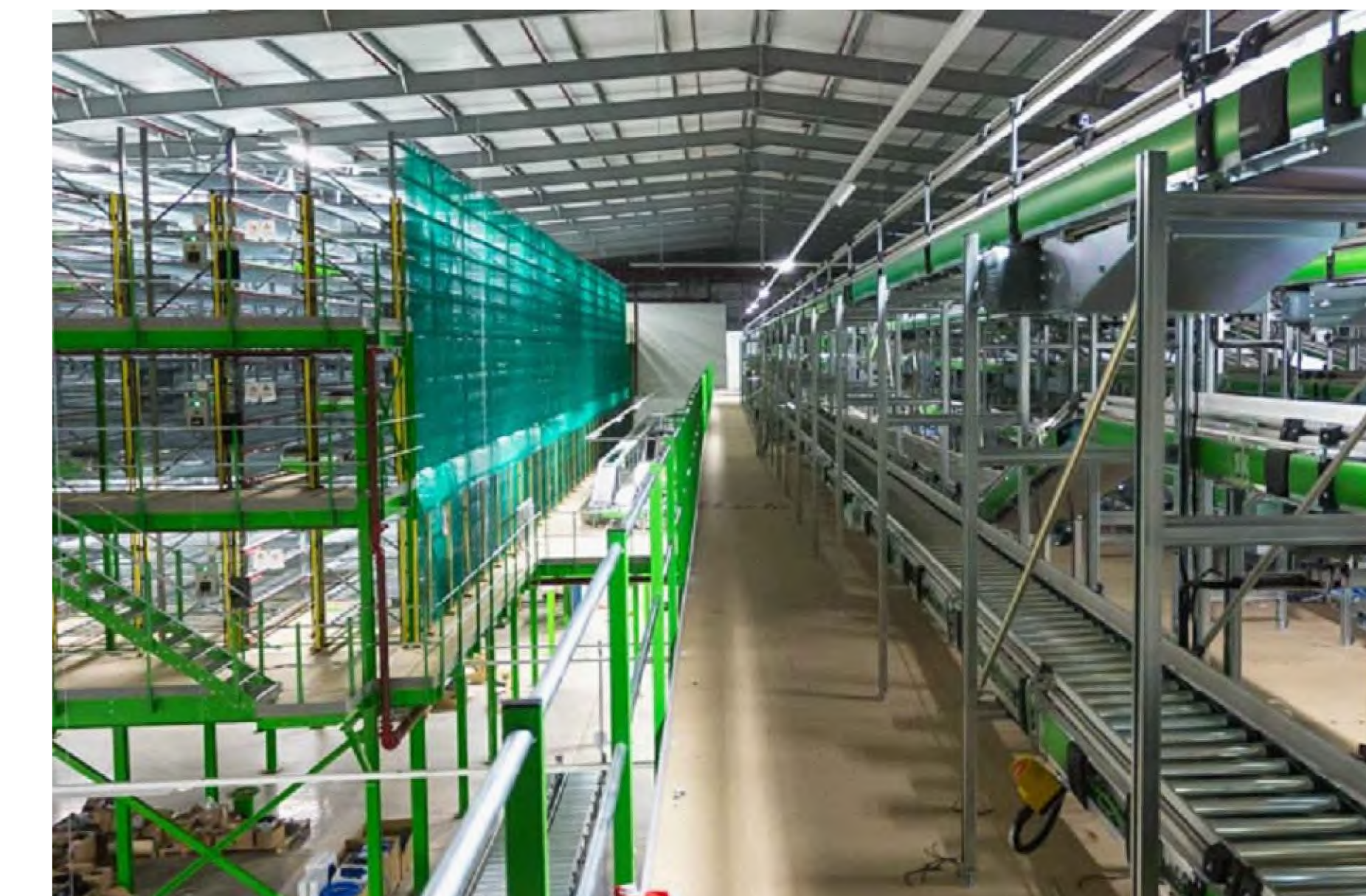
Image 2 - Mezzanine racking and automation systems
